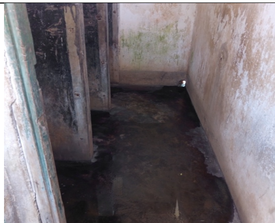
Photo 2: Girls toilet flooded with urine
