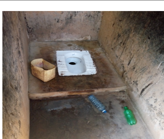
Photo 4: Plastic bottles often block the toilets
