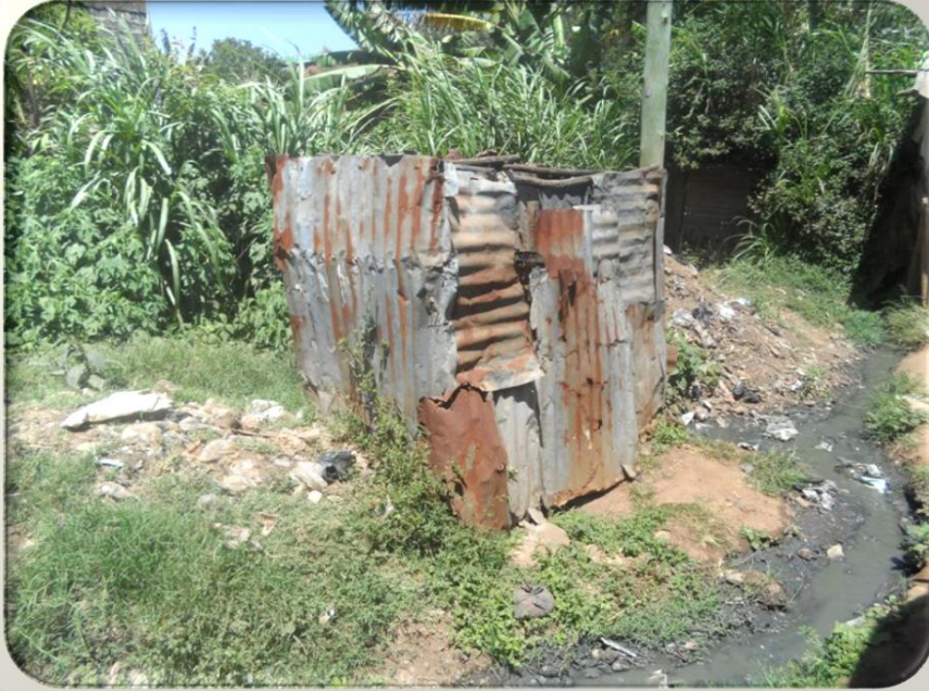
Pic: 4.4: An isolated pit latrine emitting effluents to sewer line in Mathari 4A informal settlement
