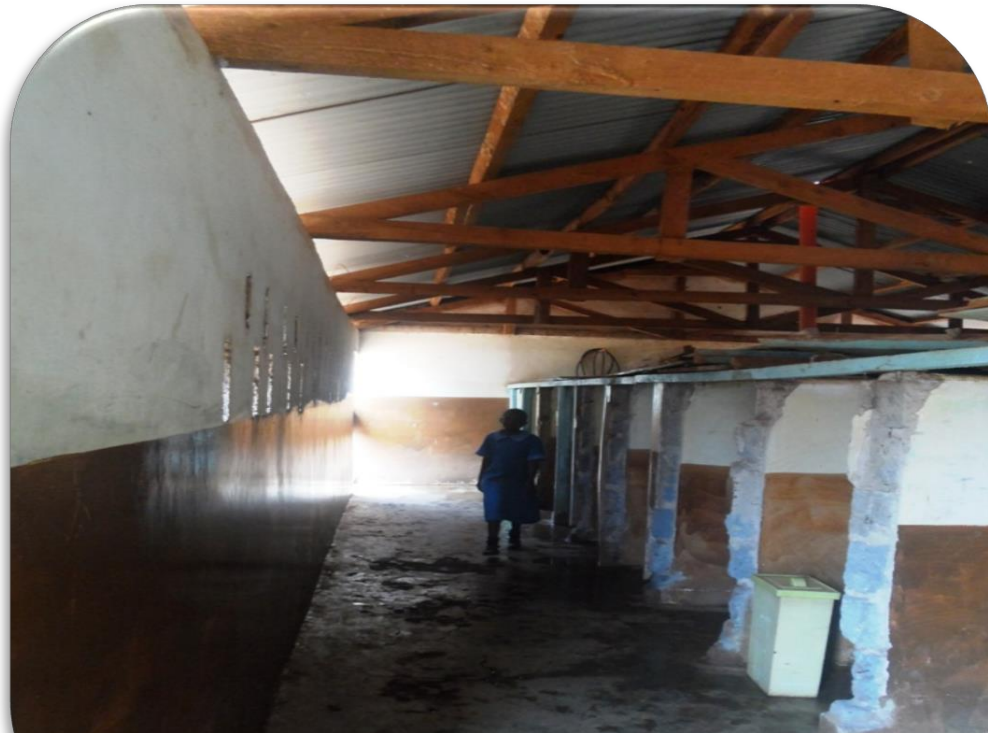
Pic 4.5: No privacy: One of the girl's sanitation facilities In Kasarani Primary School. The facility has poor lighting and lacks doors in its cubicles. The facility also has only one sanitary disposal bin.
